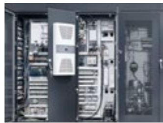
Climatized electric cabinet with easy access, isolated from heat-sources.
